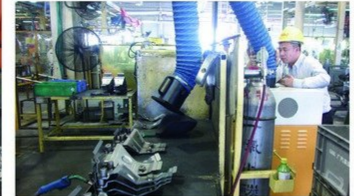
Fume extraction for the metal piece welding
