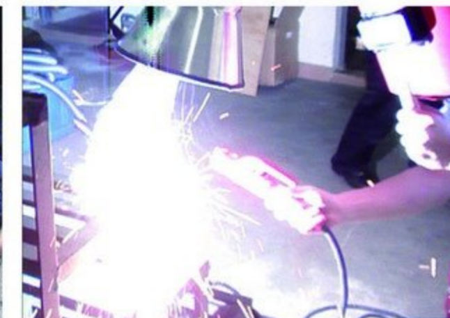
welding workshop supported fume extraction
